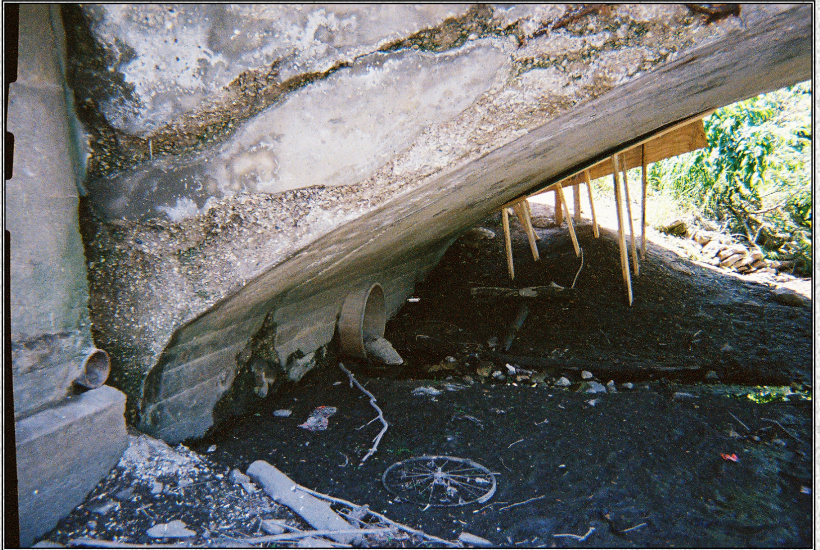
Deteriorated condition of the east abutment and spandrel arch on the original structure.
